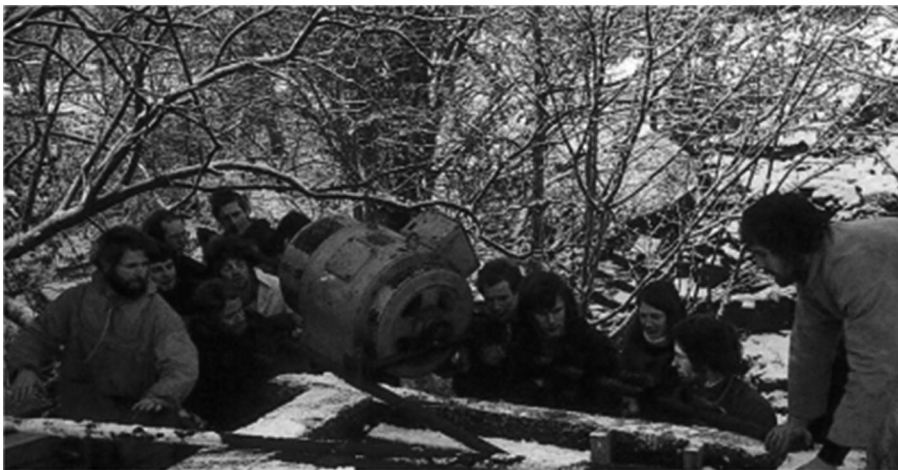
Figure 2. Installing CAT’s first AC generator onto its operating platform. Credit: Centre for Alternative Technology.
